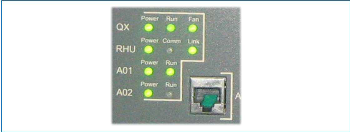
LED Indication of Normal Operation | Figure 3-26
