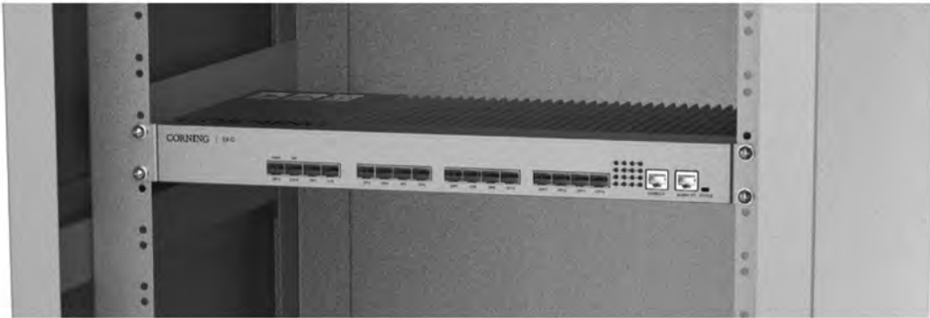
Figure 18. E3 in Rack
