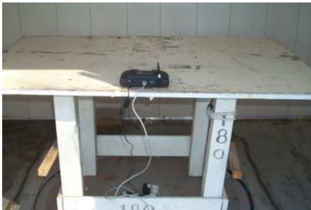
Typical Hosting I: Base Unit-Position X w/ Interior Antenna
