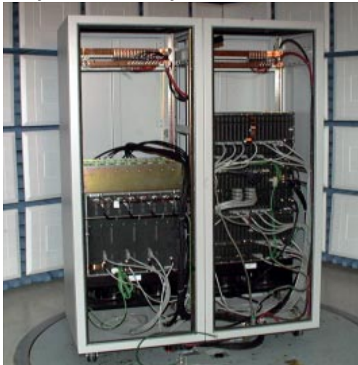
Figure 12.5 Base Configuration, Rear Panels Removed—Rear View
