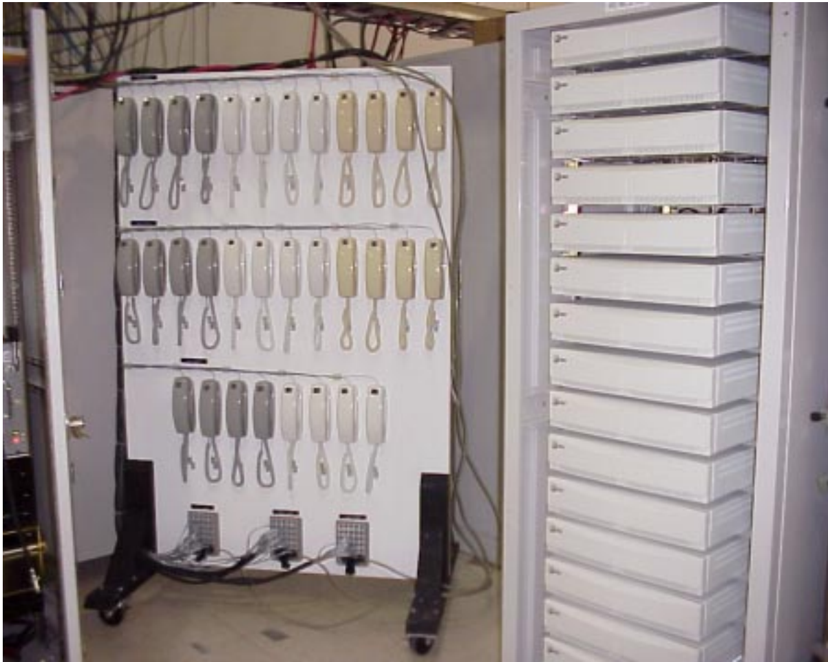
Figure 12.10 RU test rack
