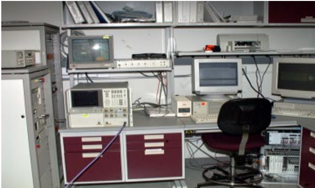
Figure 12.6 3-meter Shield Room Control Room
