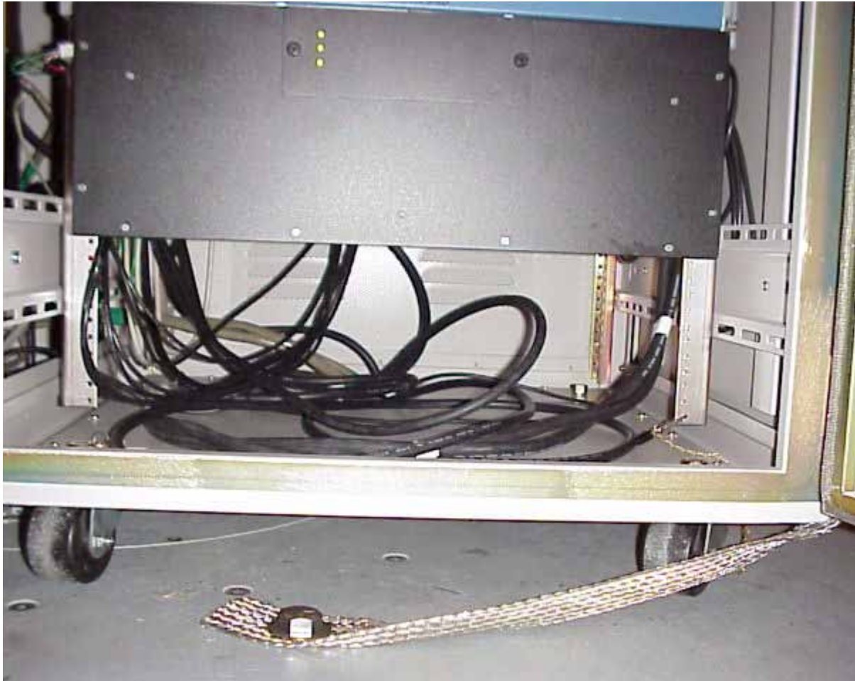
Figure 6.22—Bottom view of the PWAN Base RF Cabinet
