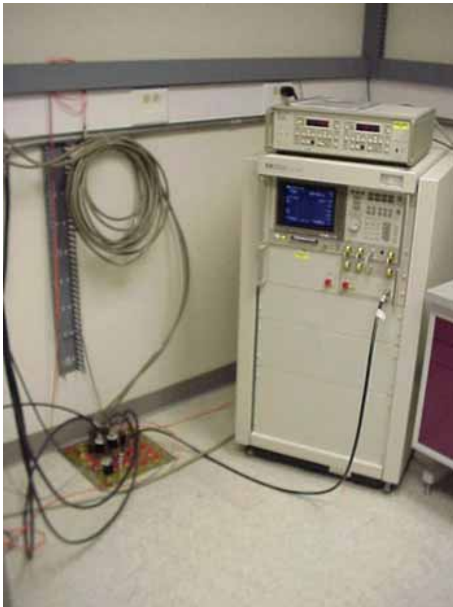
Figure 12.7—3 meter control room
