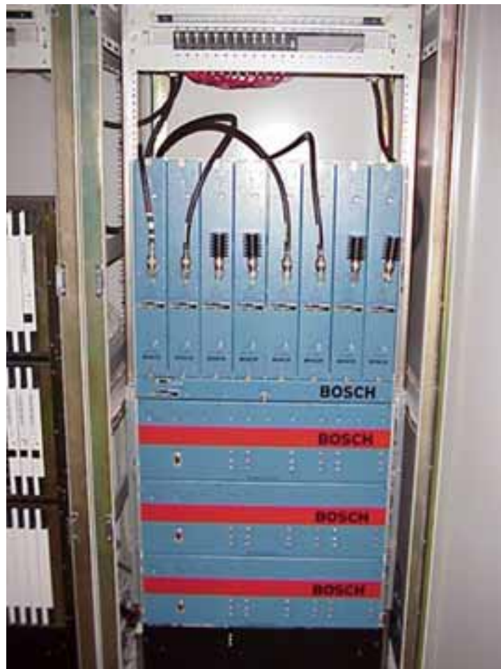
Figure 6.21—Overview of the PWAN Base RF Cabinet
