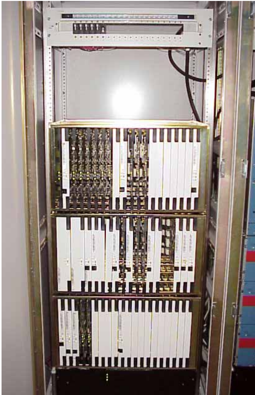
Figure 6.1— Overview of the PWAN Base Digital Cabinet.
