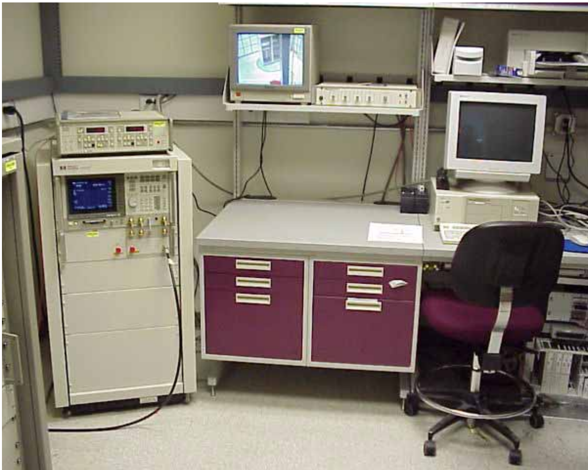
Figure 12.6—3 meter shield room control room
