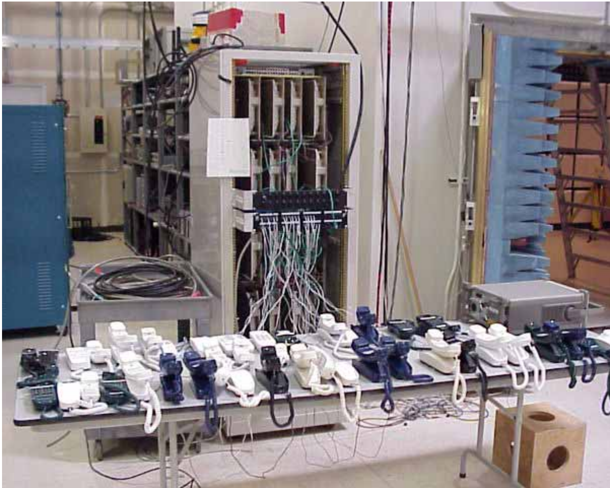
Figure 12.10—RU test rack
