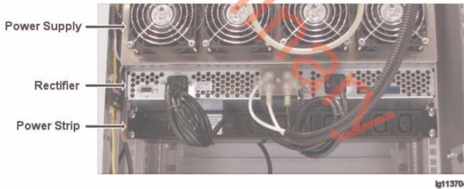
Figure 1-9: Power Supply, Rectifier, and Power Strip Rear
