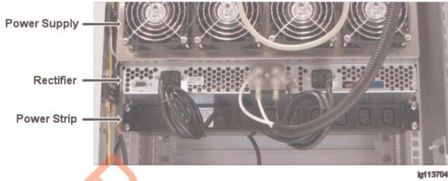
Figure 2-2: Power Supply, Rectifier, and Power Strip Rear
