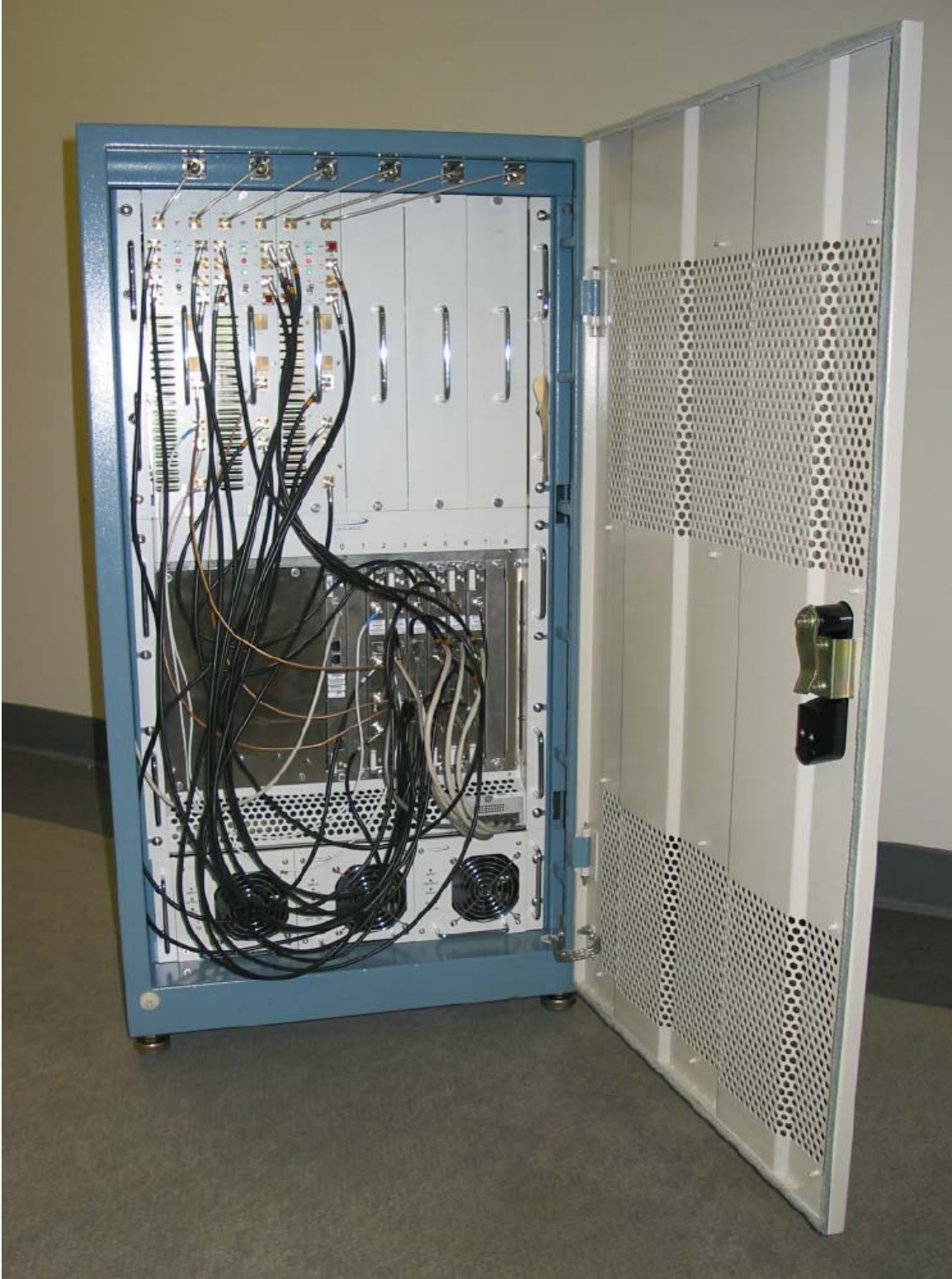
Base Station UltraWAVE BTS, AUAC85, Front View
