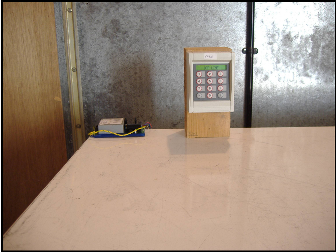
AC Powerline Conduction
