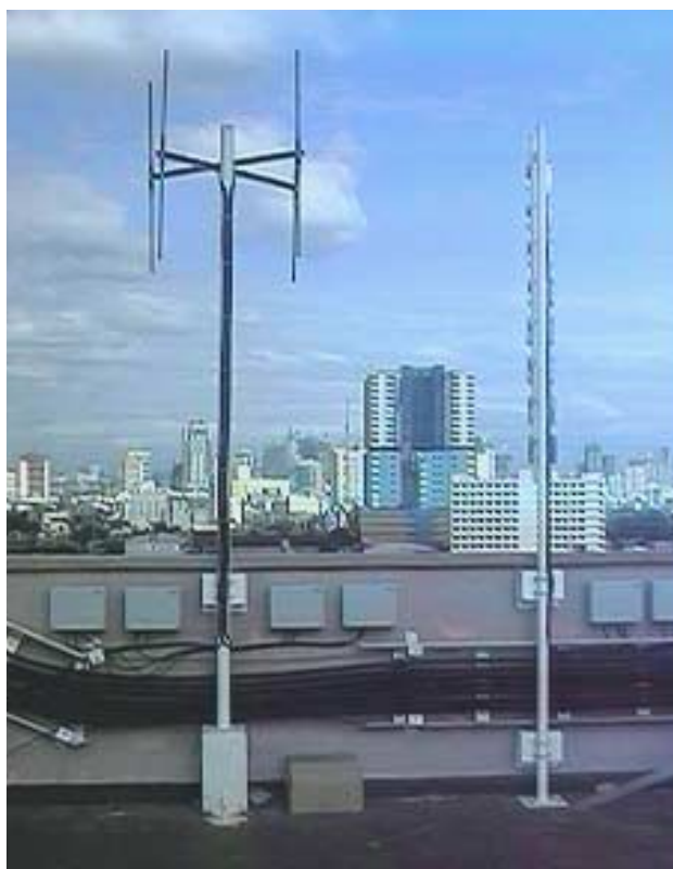
Figure 5-8: Outdoor 10mW RPs installed on rooftop
