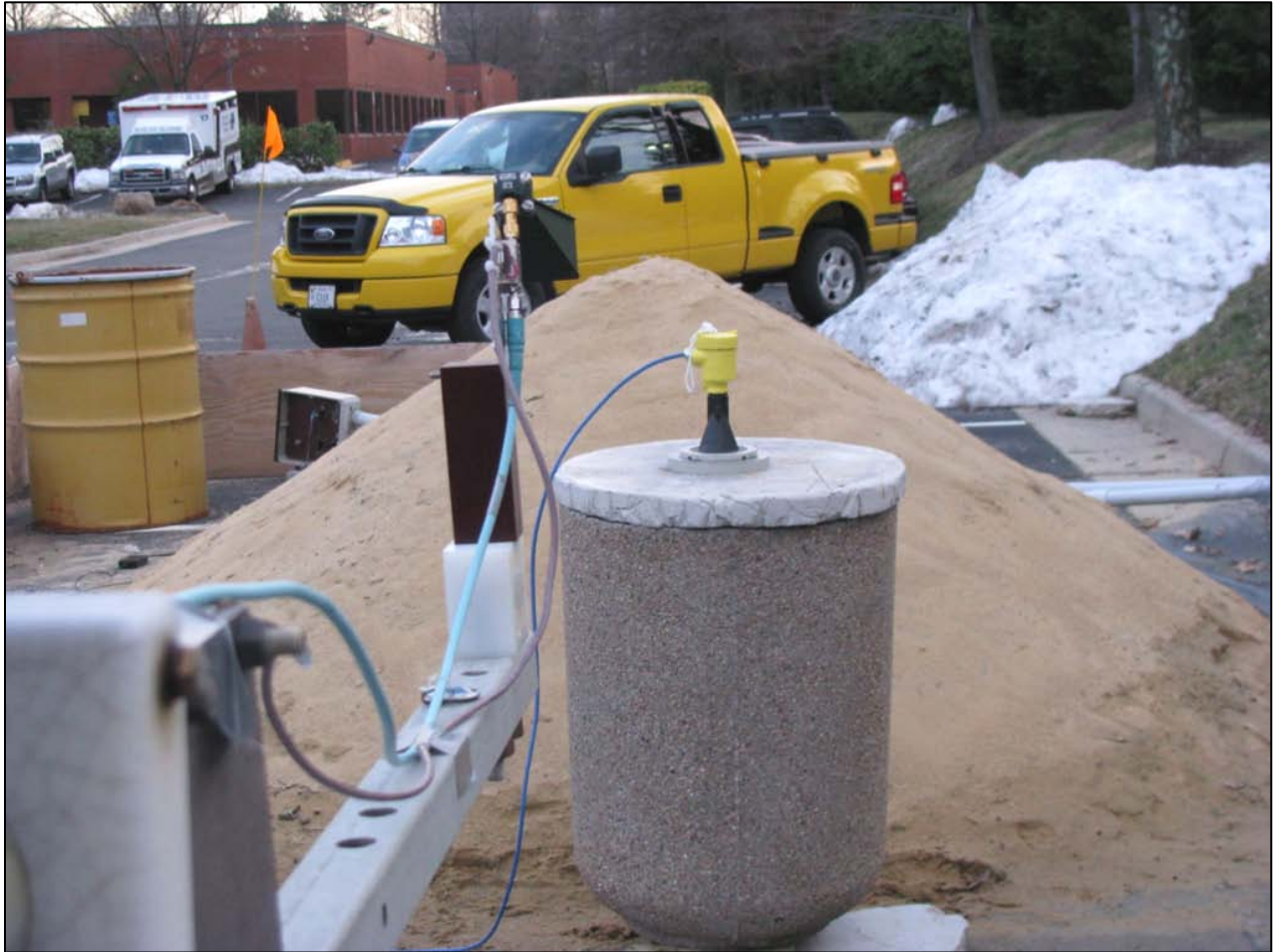
Photograph 29: 80mm Plastic Antenna Front View Concrete Tank
