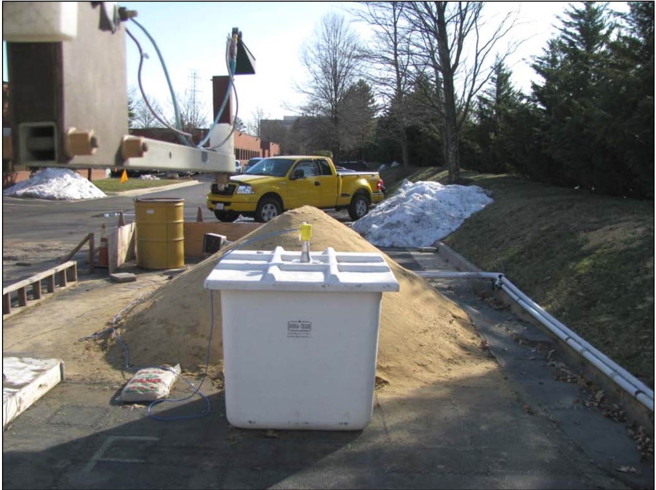
Photograph 41: 75mm Metal Antenna Front View Fiberglass Tank
