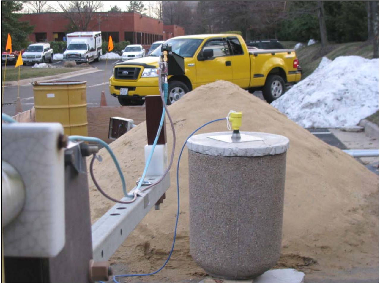
Photograph 31: 1/2" Stub Antenna Front View Concrete Tank
