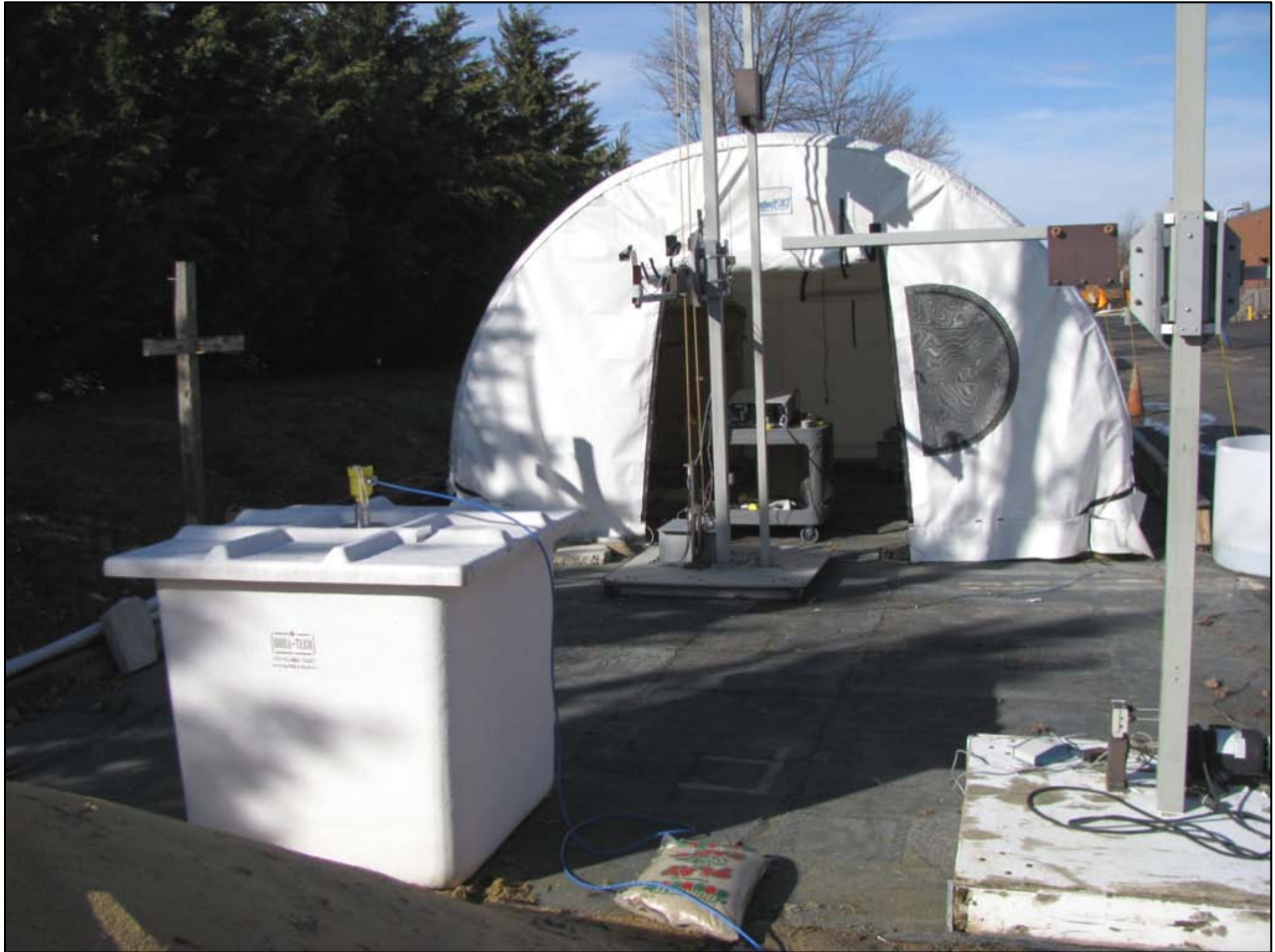
Photograph 44: 48mm Metal Antenna Rear View Fiberglass Tank
