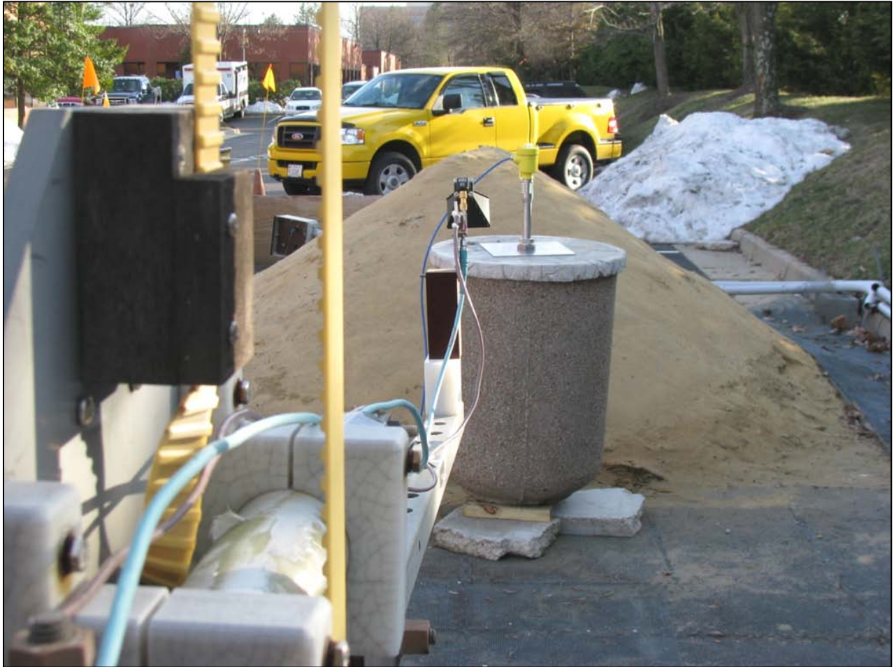
Photograph 34: 1/2" Standpipe Antenna Rear View Concrete Tank
