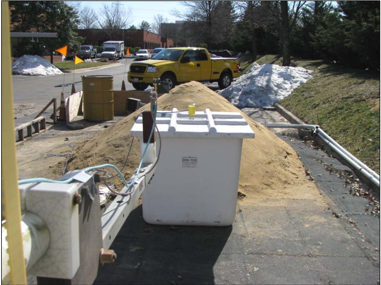
Photograph 39: 40mm Antenna Front View Fiberglass Tank
