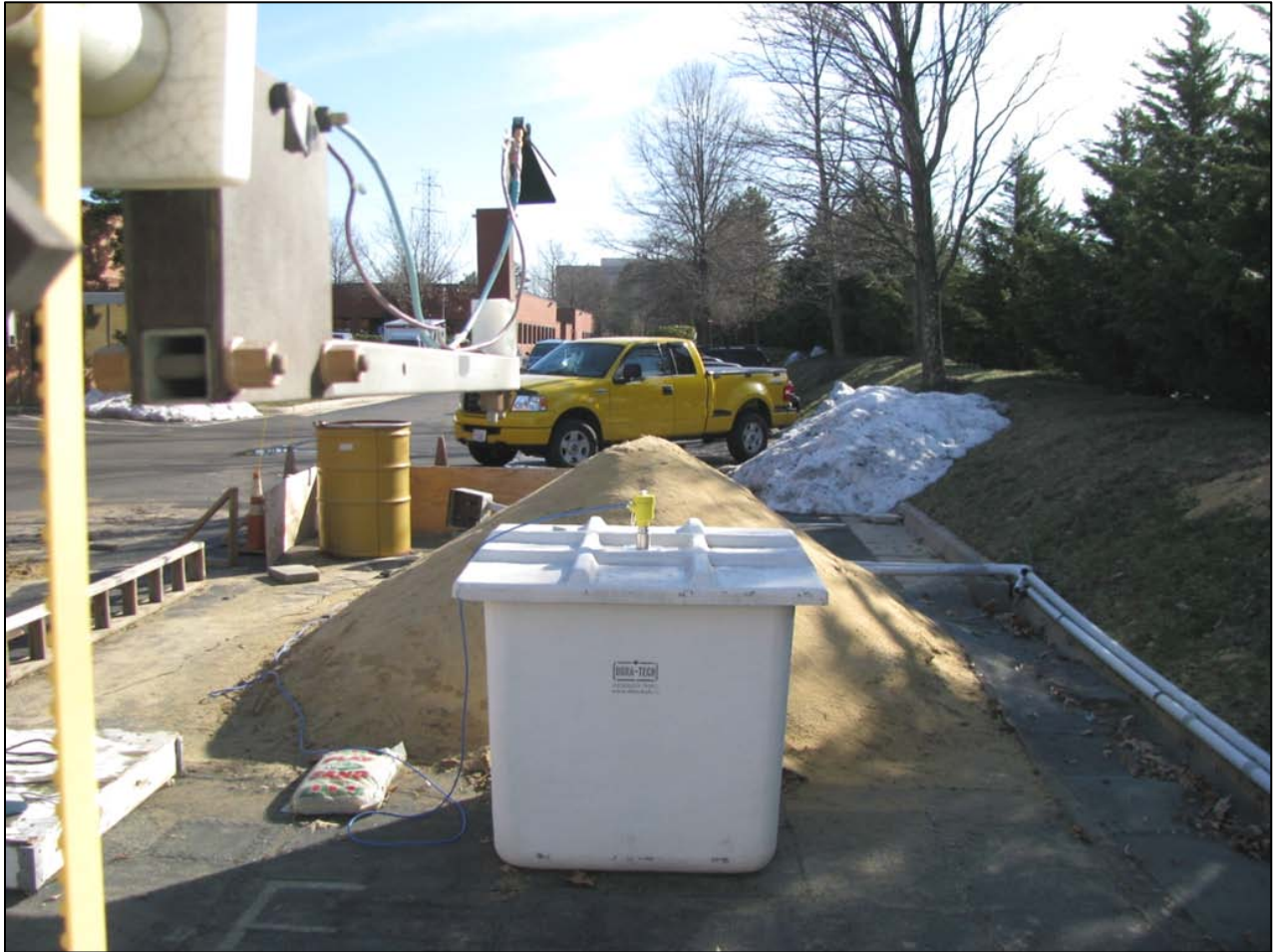
Photograph 43: 48mm Metal Antenna Front View Fiberglass Tank
