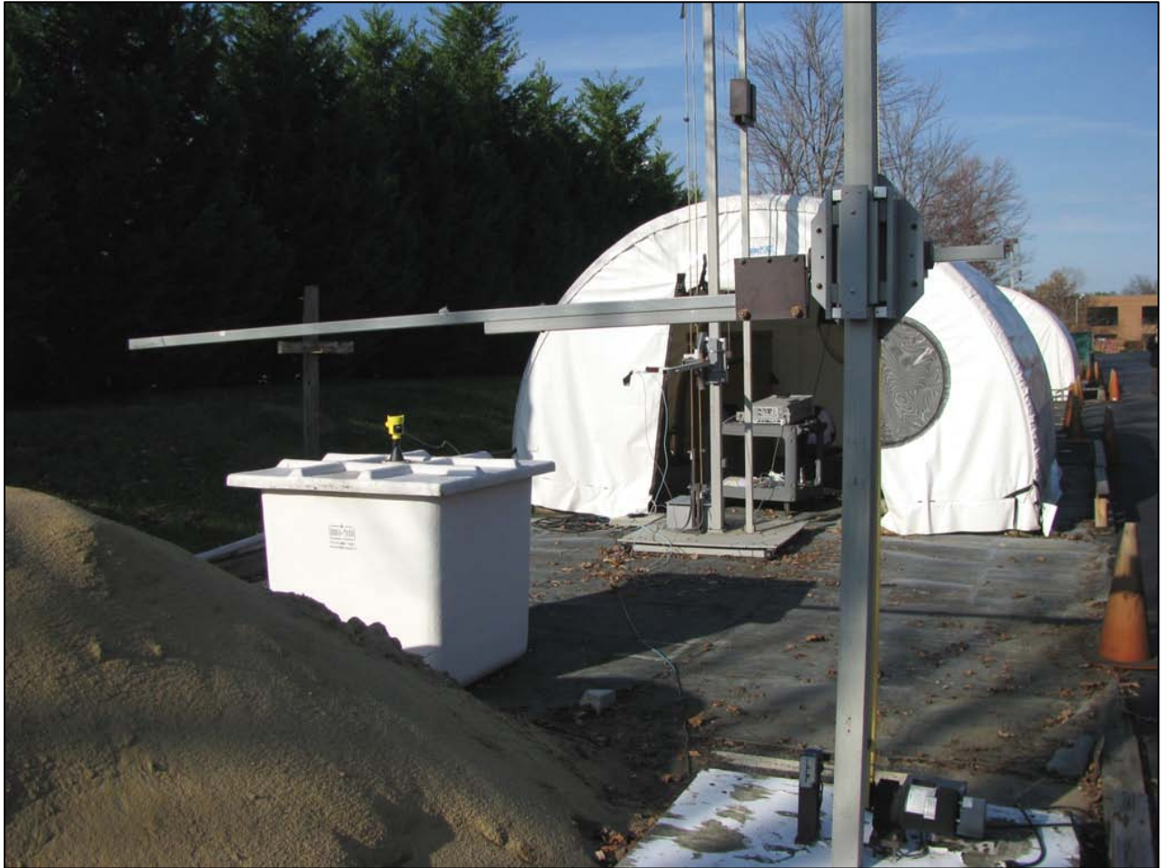
Photograph 46: 80mm Plastic Antenna Rear View Fiberglass Tank
