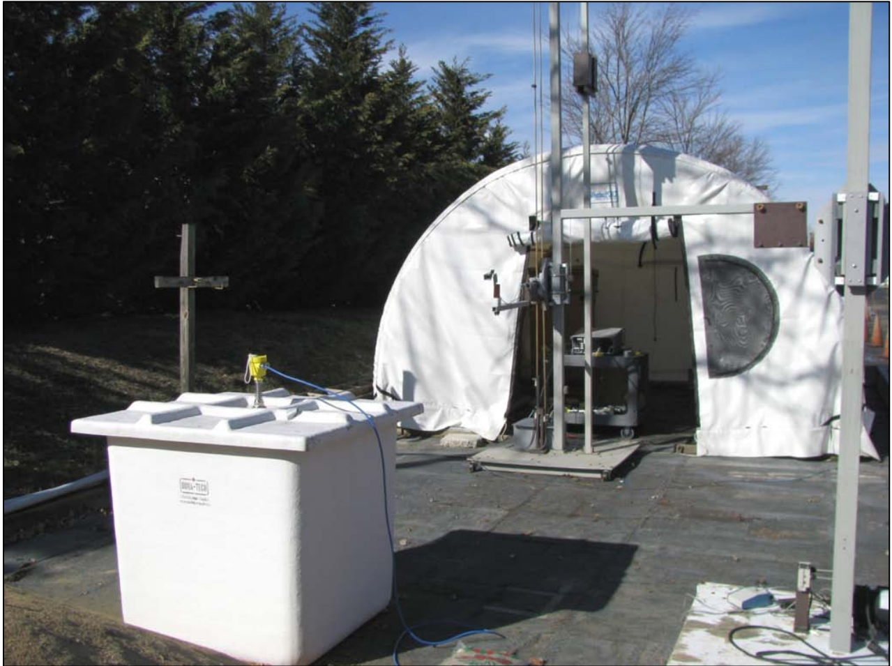
Photograph 50: 1/2" Standpipe Antenna Rear View Fiberglass Tank
