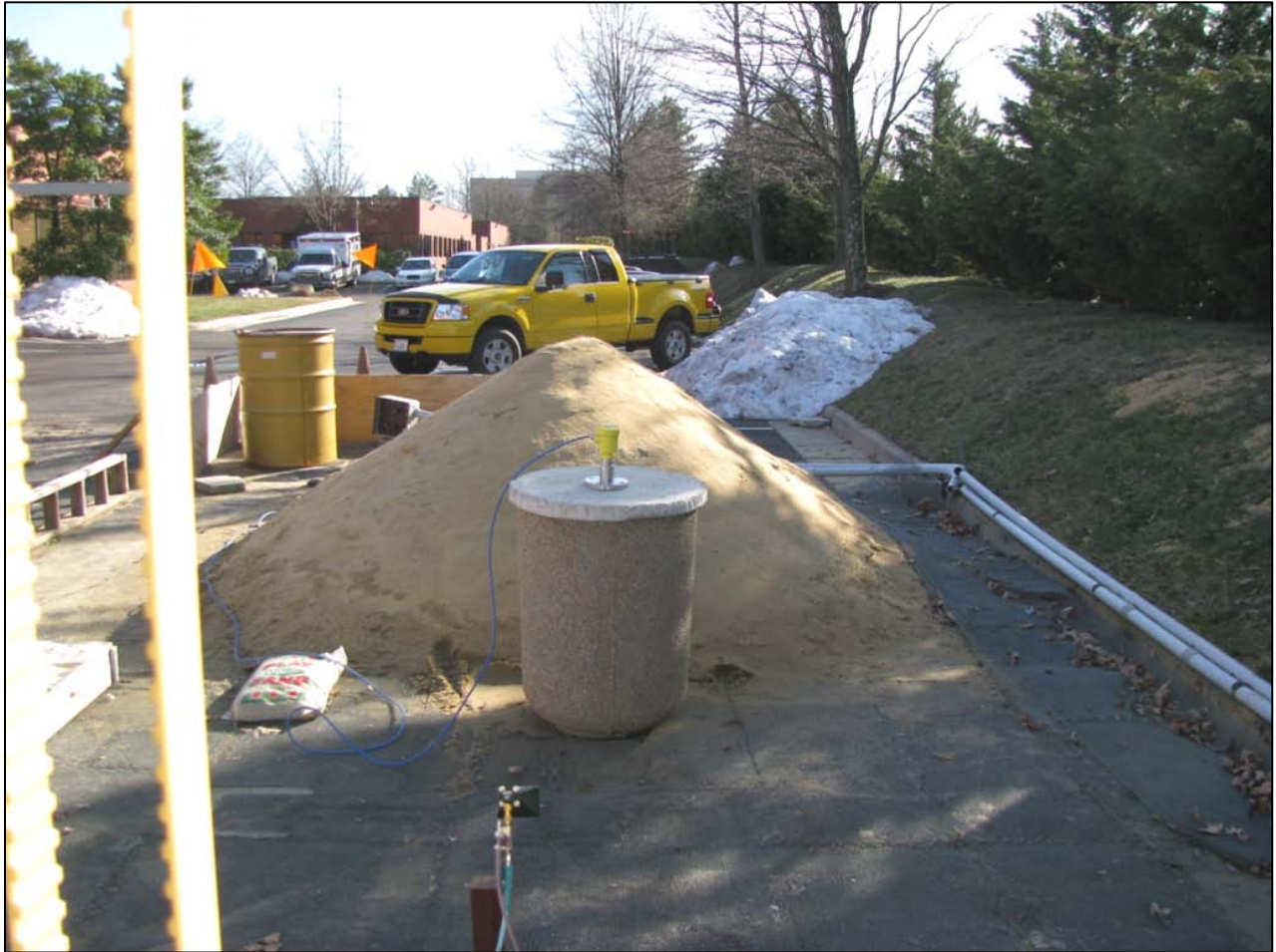
Photograph 27: 48mm Metal Antenna Front View Concrete Tank
