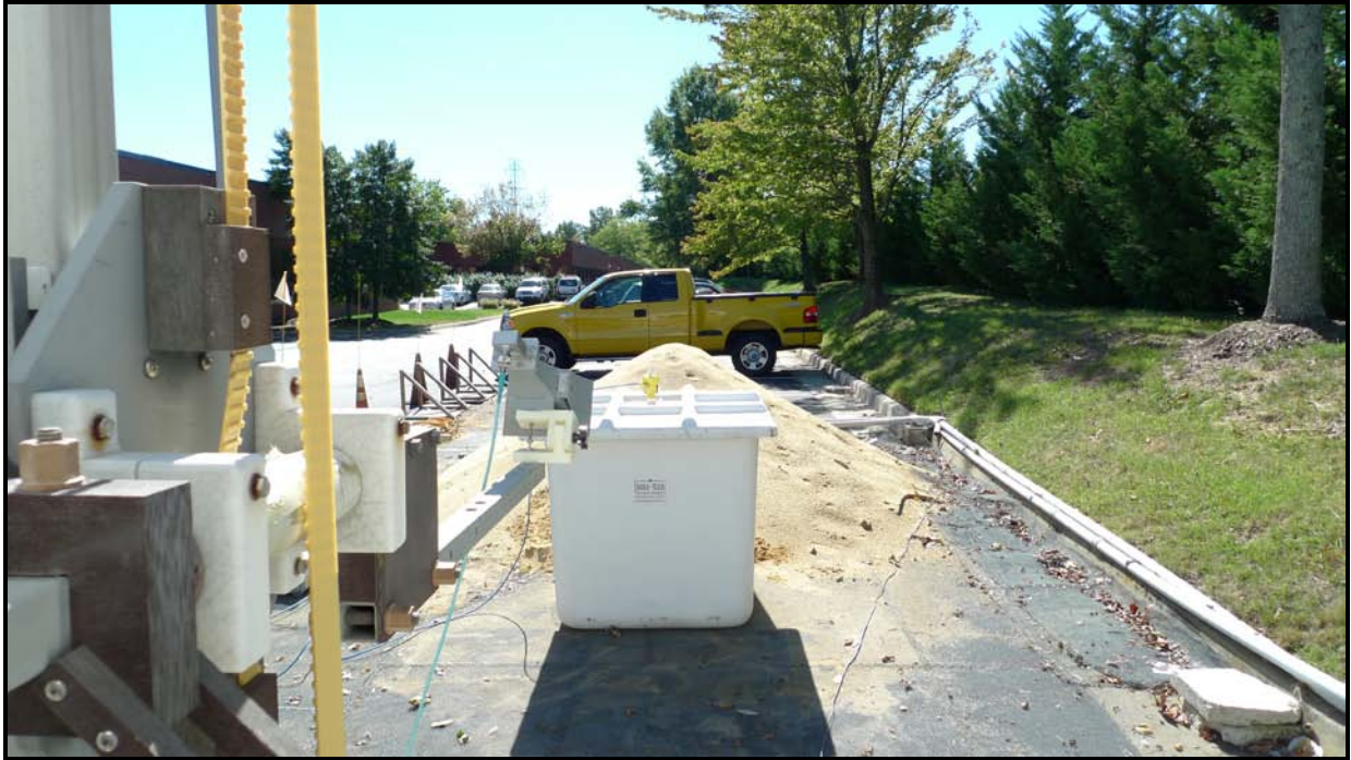
Photograph 25: 50mm Rod Antenna Front View Fiberglass Tank
