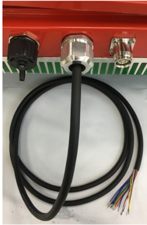
Figure 5-5: Alarm Relay Cable Connected to Signal Booster
