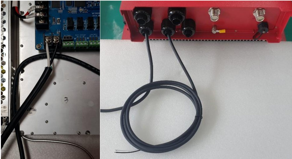
Figure 5-10: Battery Cable Connected to Signal Booster
