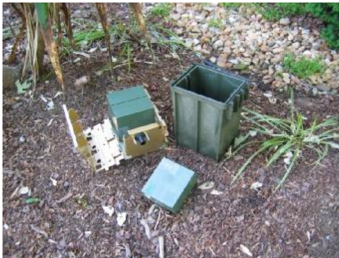
Figure 2-2: The Battery Box contains the housing that the batteries plug into
