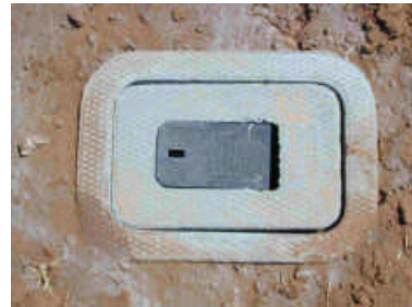
Concrete Pit w. concrete cover and metal lid
