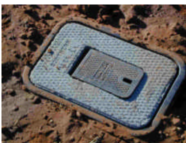
Plastic Pit w. concrete cover and metal lid
