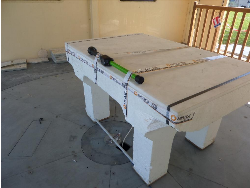
Position 3 supplied by battery
