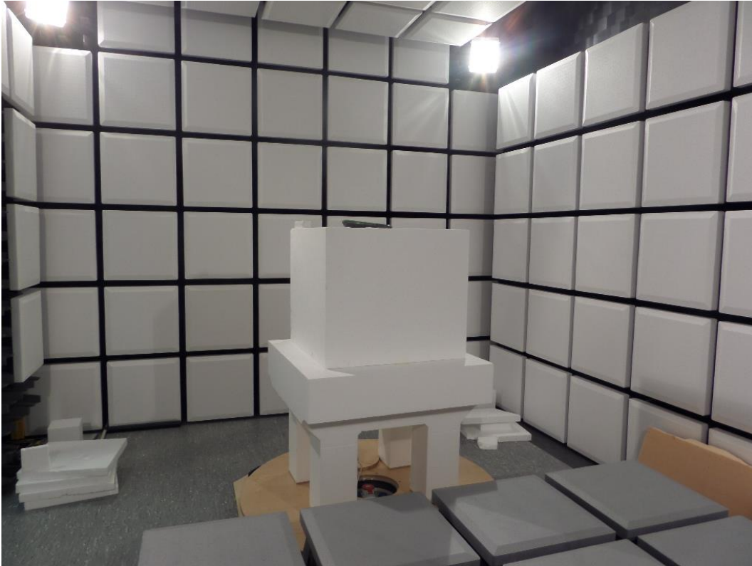
Anechoic room – Position 2 supplied by battery
