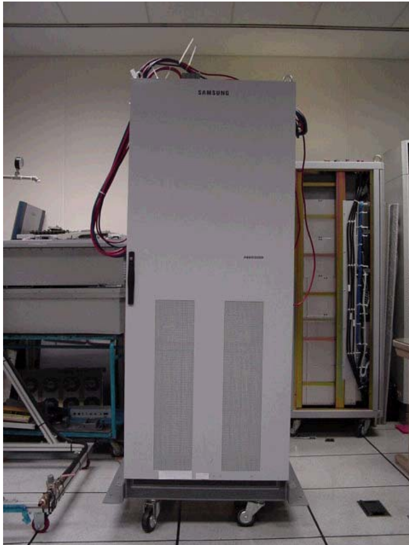
Photos of Indoor BTS
