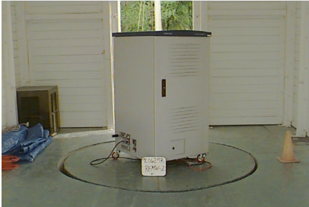
Photo 2 - Outdoor Mini-BTS FRONT VIEW
