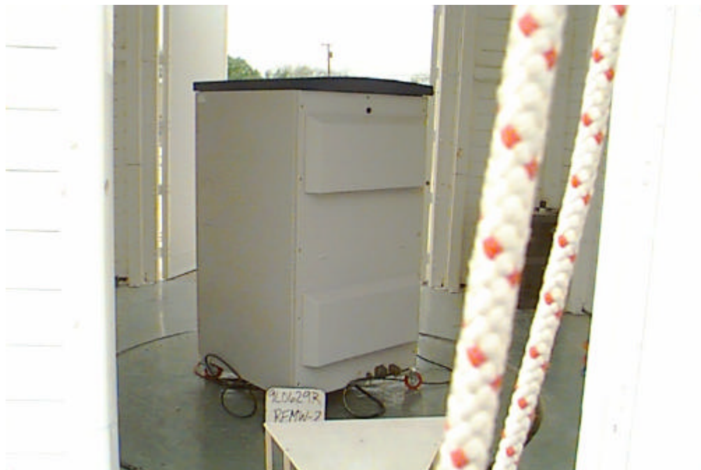
Photo 1 - Indoor Mini-BTS REAR VIEW
