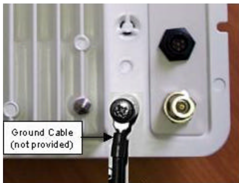
Figure 7 – Detail Showing Ground Cable Connection (this provides maximum lightning protection)
