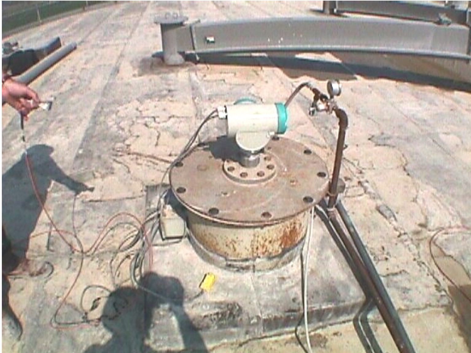
The Siemens Milltronics SITRANS LR mounted on top of the mouth of the Concrete Tank
