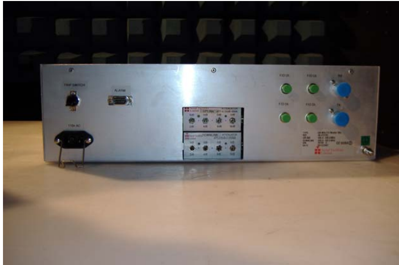
Fibre Optic Tray Rear Overview
