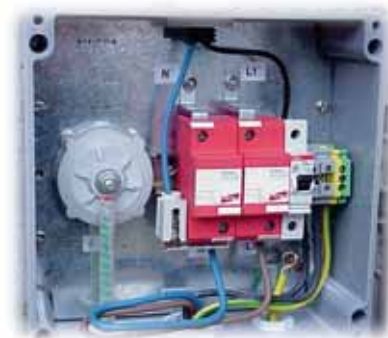
Figure 3-4: Protective device installed in connection with the power supply
