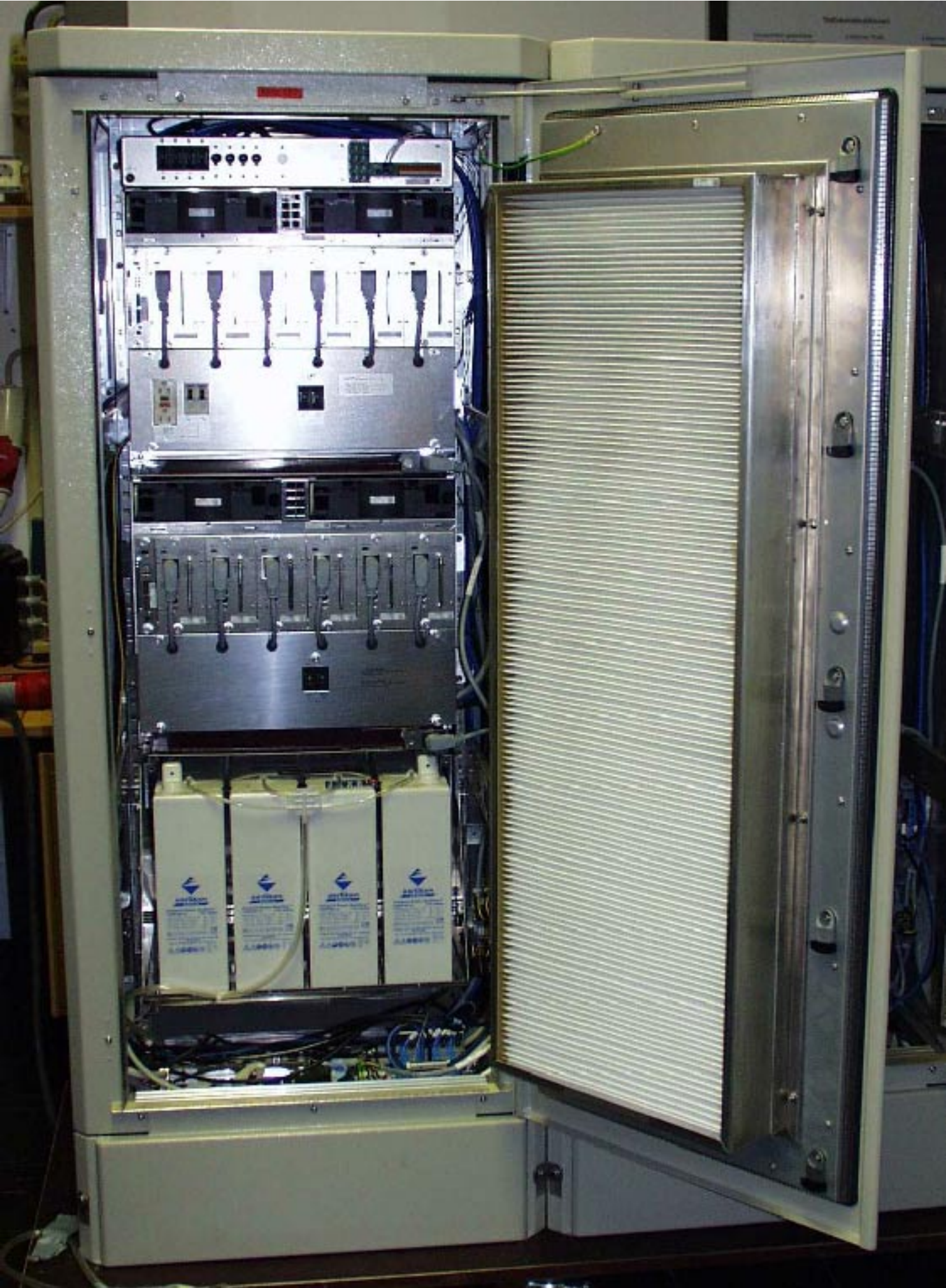
BS-241U Service shelter - Front door open
