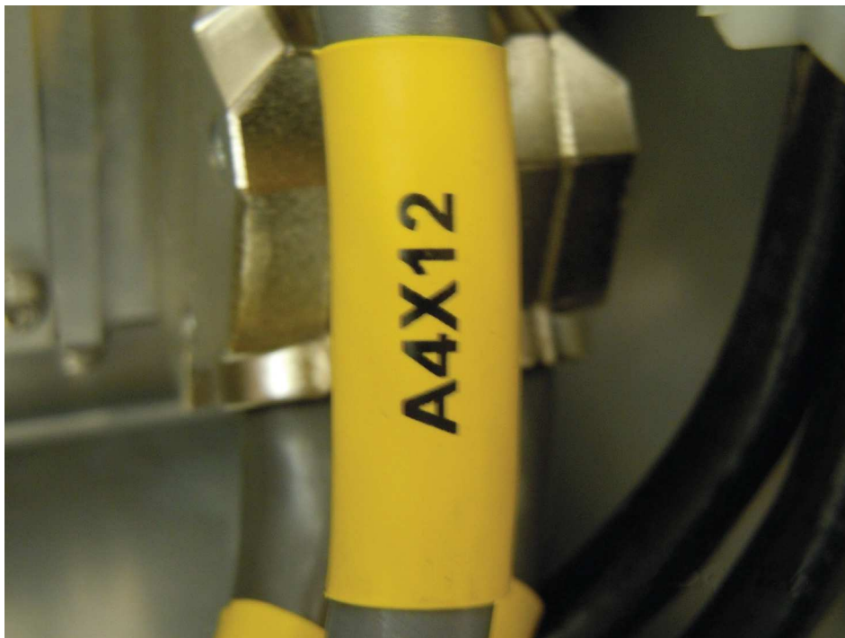
Fig. 7.4 Marking, other cables
