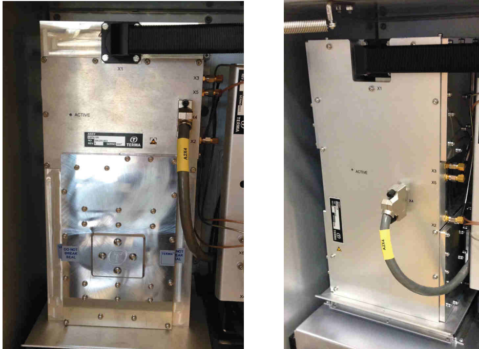
Fig. 4.7 SSPA modules - 50 W left and 200 W to the right
