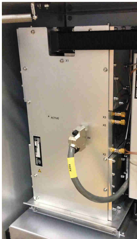
Fig. 3.2 200 watt SSPA with 4 x 50 watt PA modules
