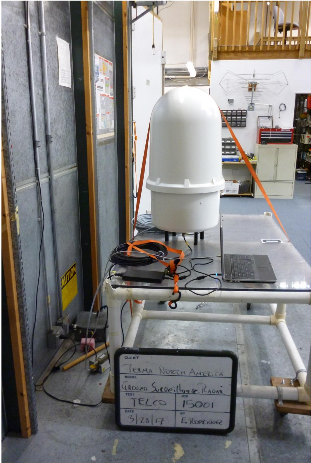
CE telco side 2
