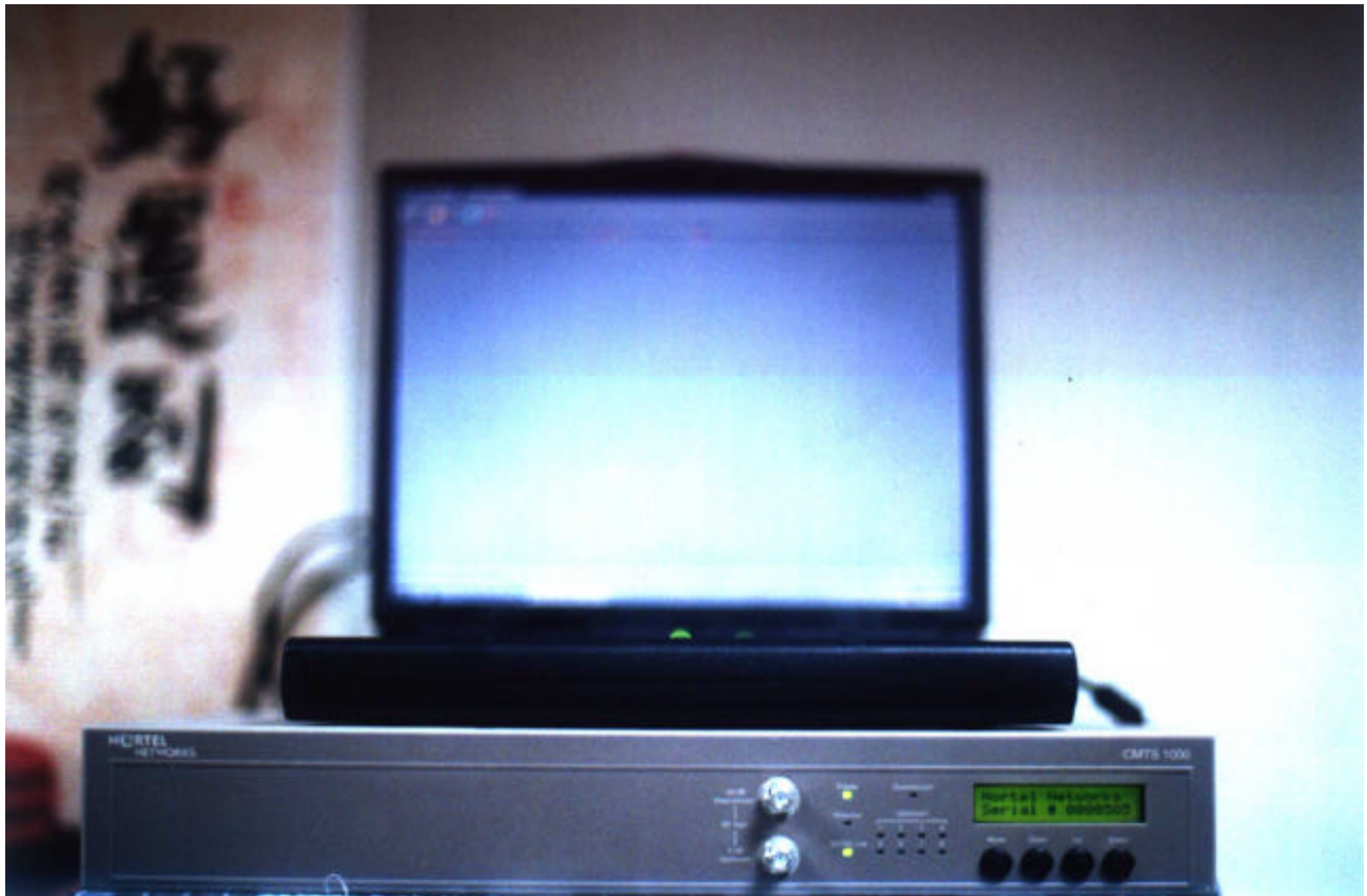
Cable Modem Head End
