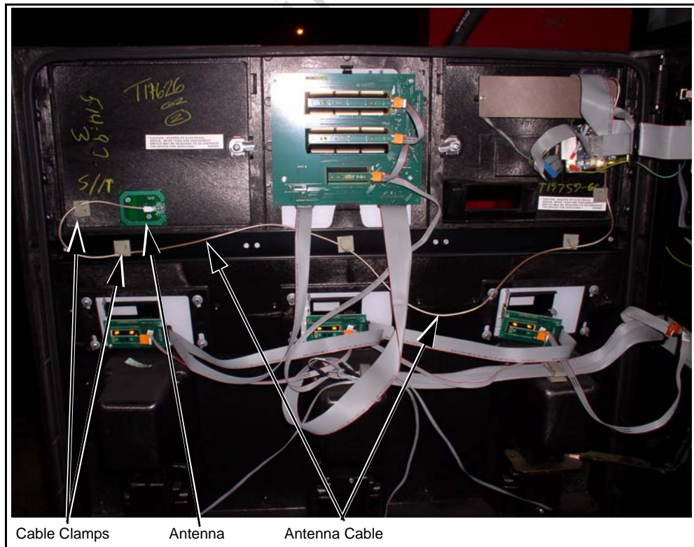
Figure 31: Cable Properly Dressed from the Antenna to the Card Reader (Looking at the Rear of the Right Door with the Door Closed)
