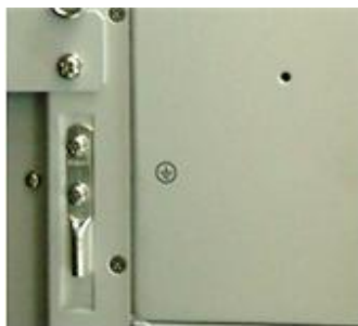
Figure 4-2 Ground Cable Connection
