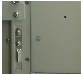
Figure 4-2 Ground Cable Connection
