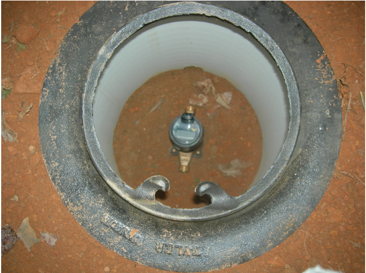
Figure 1: Radiated Emissions - Pit Installation
