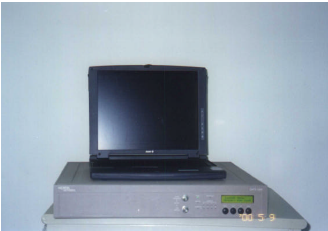
Cable Modem Head End
