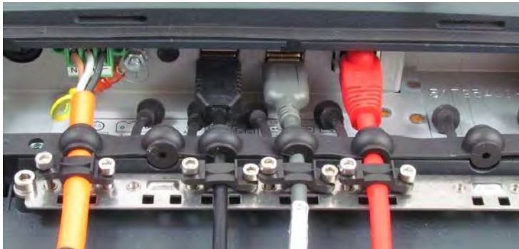
Fig. 12.6: Ethernet cable on the connector panel; secured to the strain relief rail
