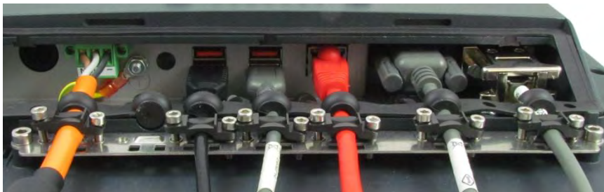
Fig. 12.7: COM cable on the connector panel; secured to the strain relief rail
