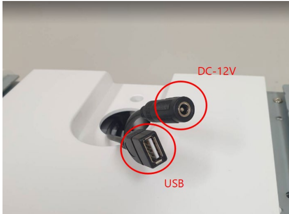
Power cable and control USB cable.
