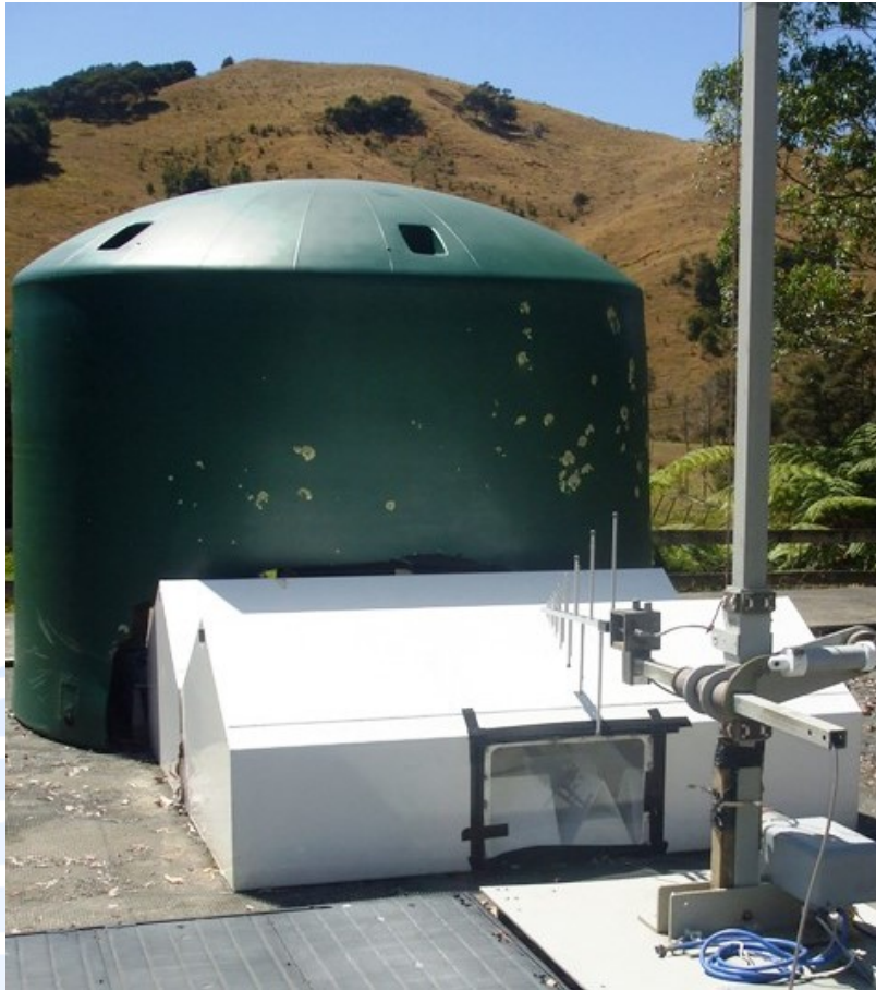
Test shed showing the use of a log periodic antenna
