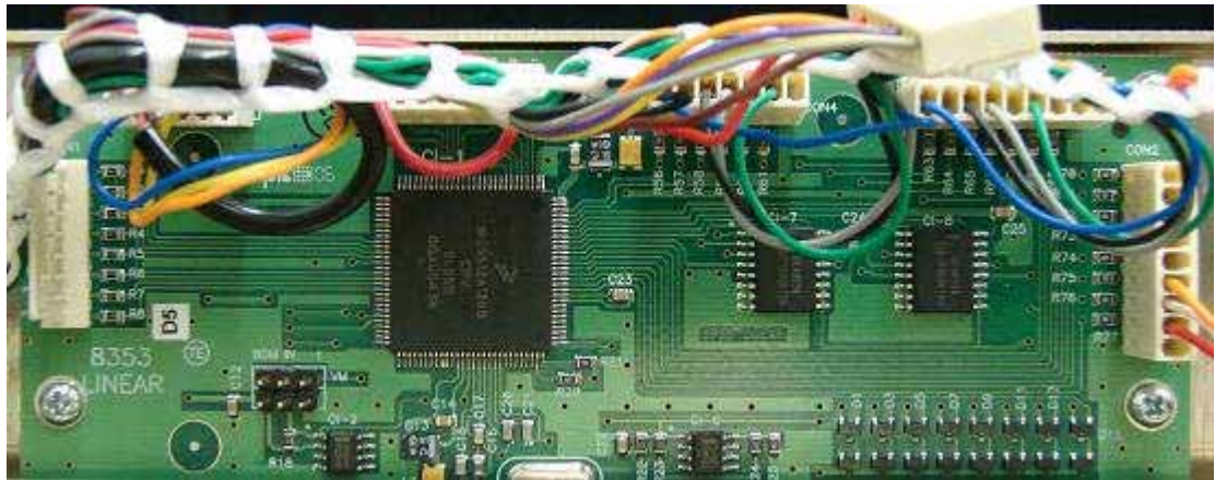
FIG. 5.7: Board CIM3452 installed on GAV4445 at bottom side, lateral right panel
