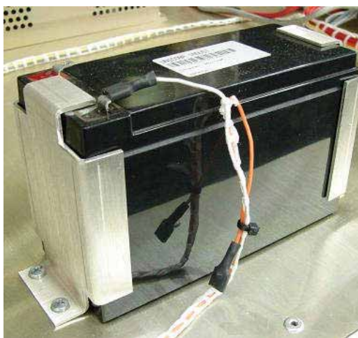
Fig.7.10: 12V/7AH Battery – shown with + cable disconnected
