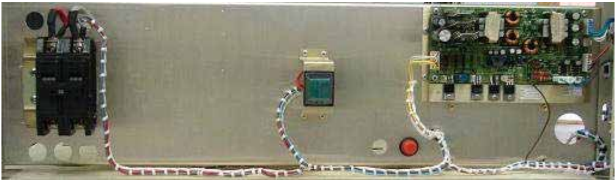
Fig.7.1: Energy Distribution – Bipolar Main Breaker on left, manual starter on the center and module 4147 – battery charger.
