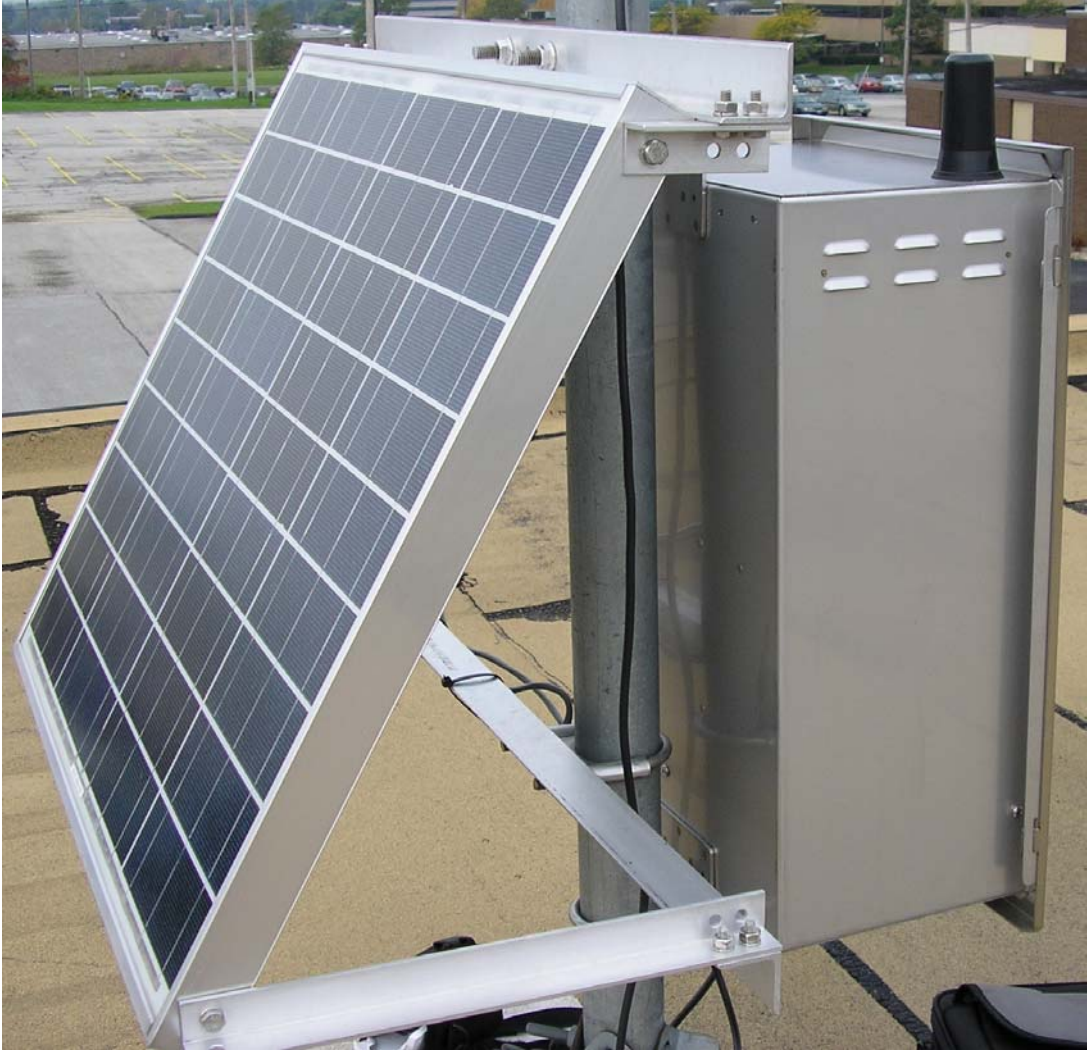
Back view and solar panel attached.
