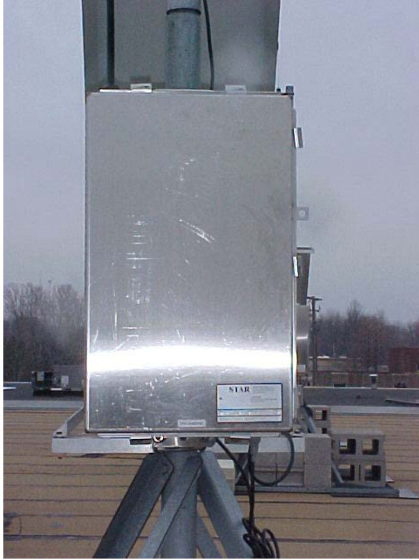
Front View on DCU
