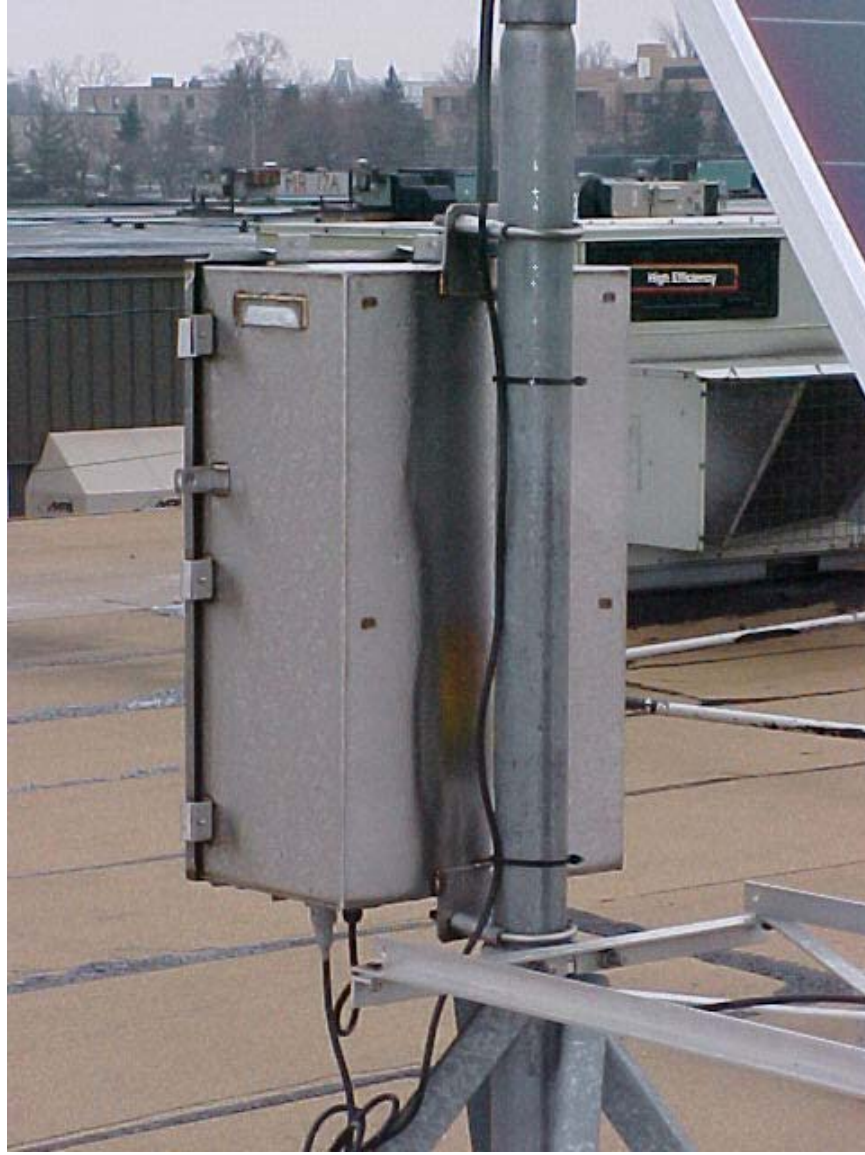
Back View on DCU
