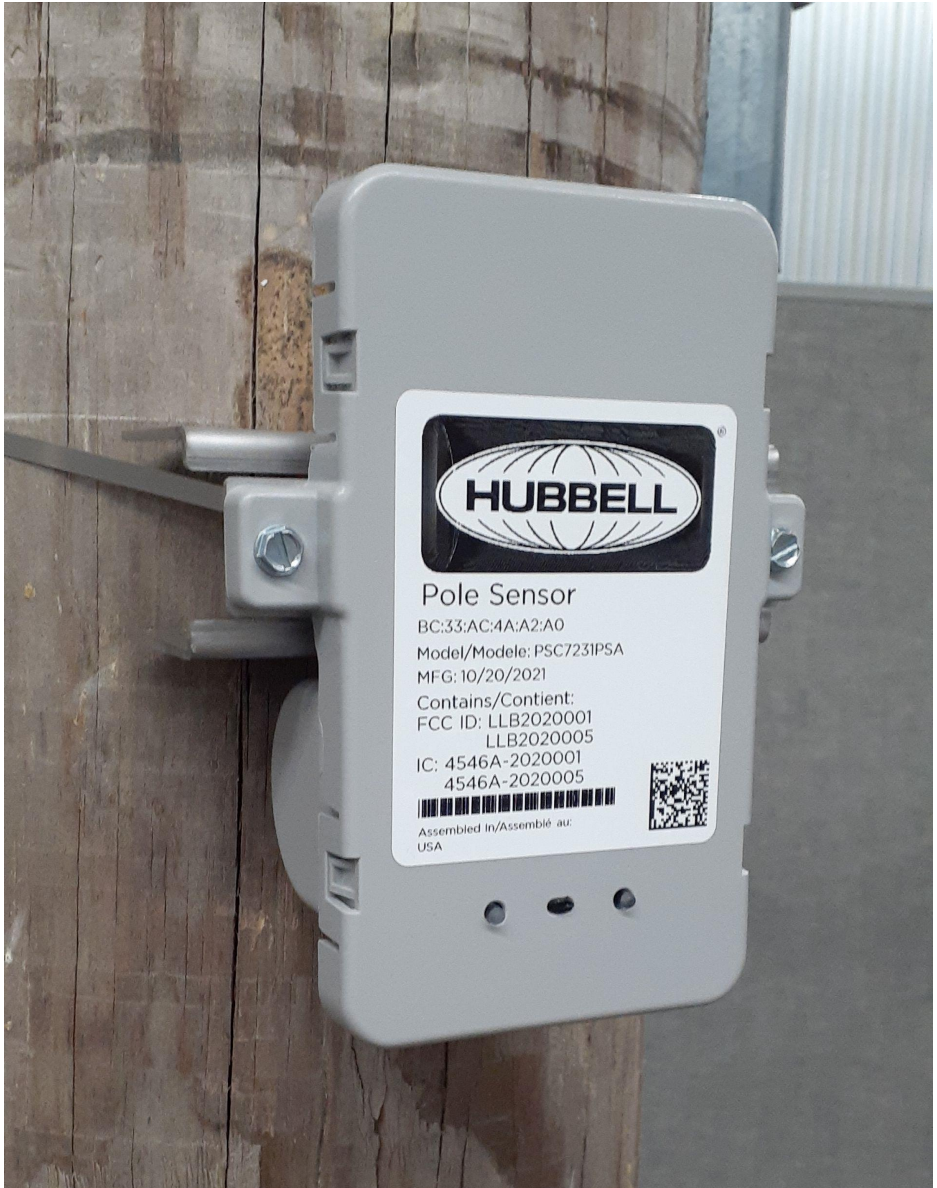
Pole Sensor installed
