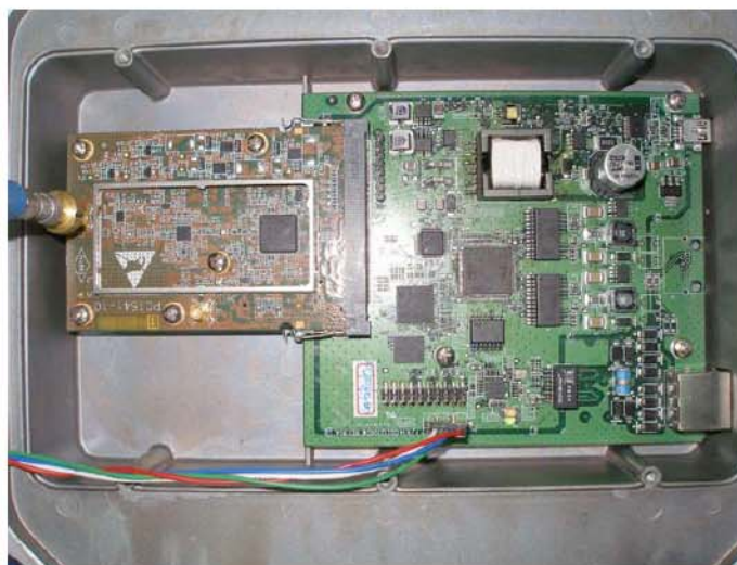
Photo #4. Outdoor unit. Internal view.
