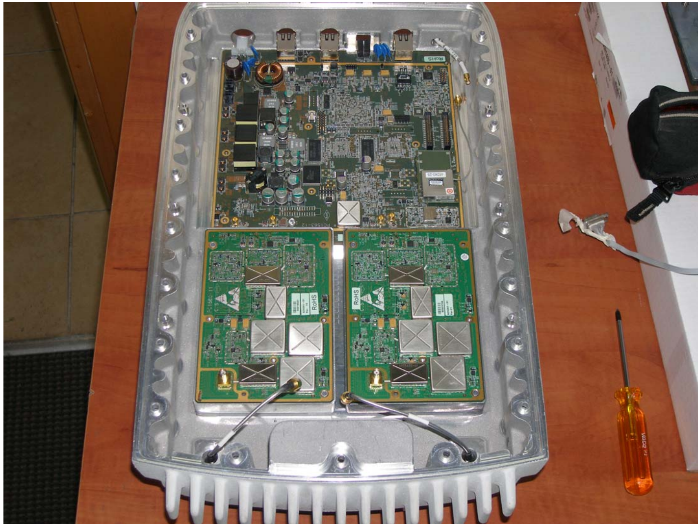
Photo9. Digital card and two radio modules CS view
