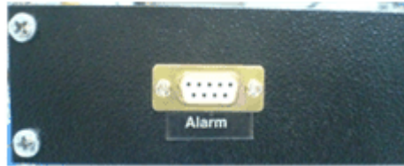
Figure 9: UDC Alarm Output
