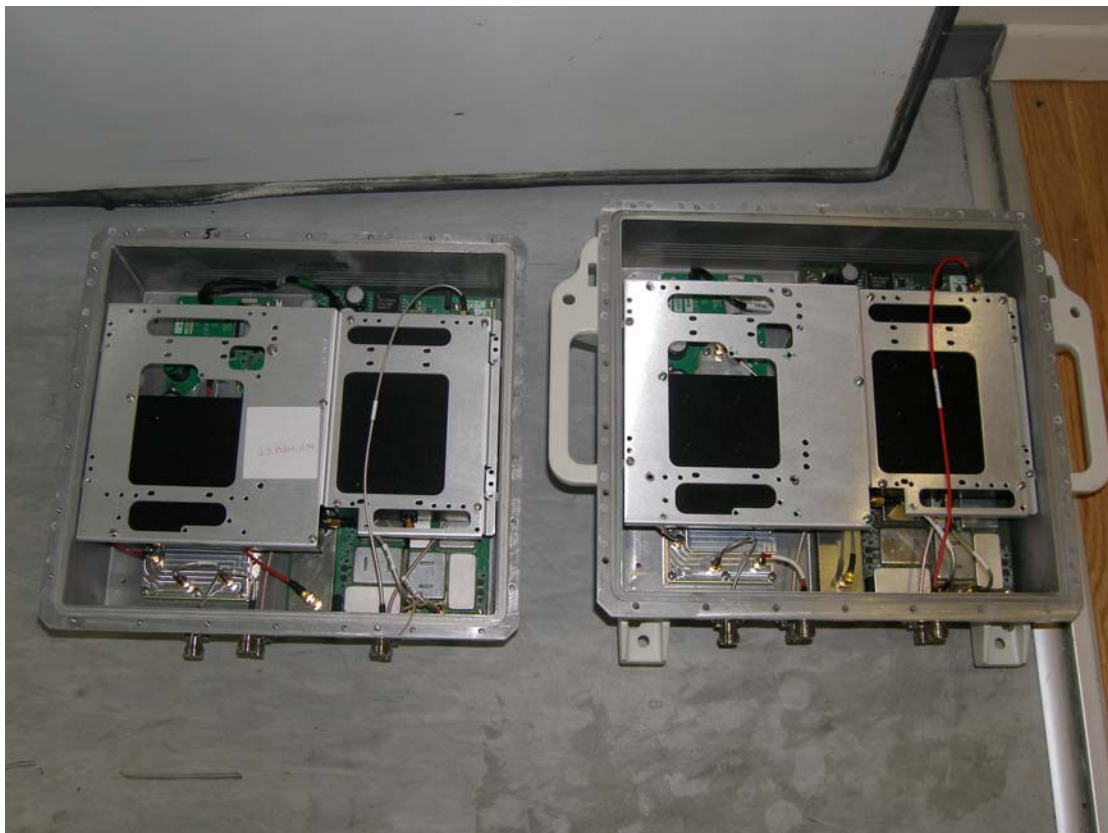
Photo4. ODU Radio open , two half sections
