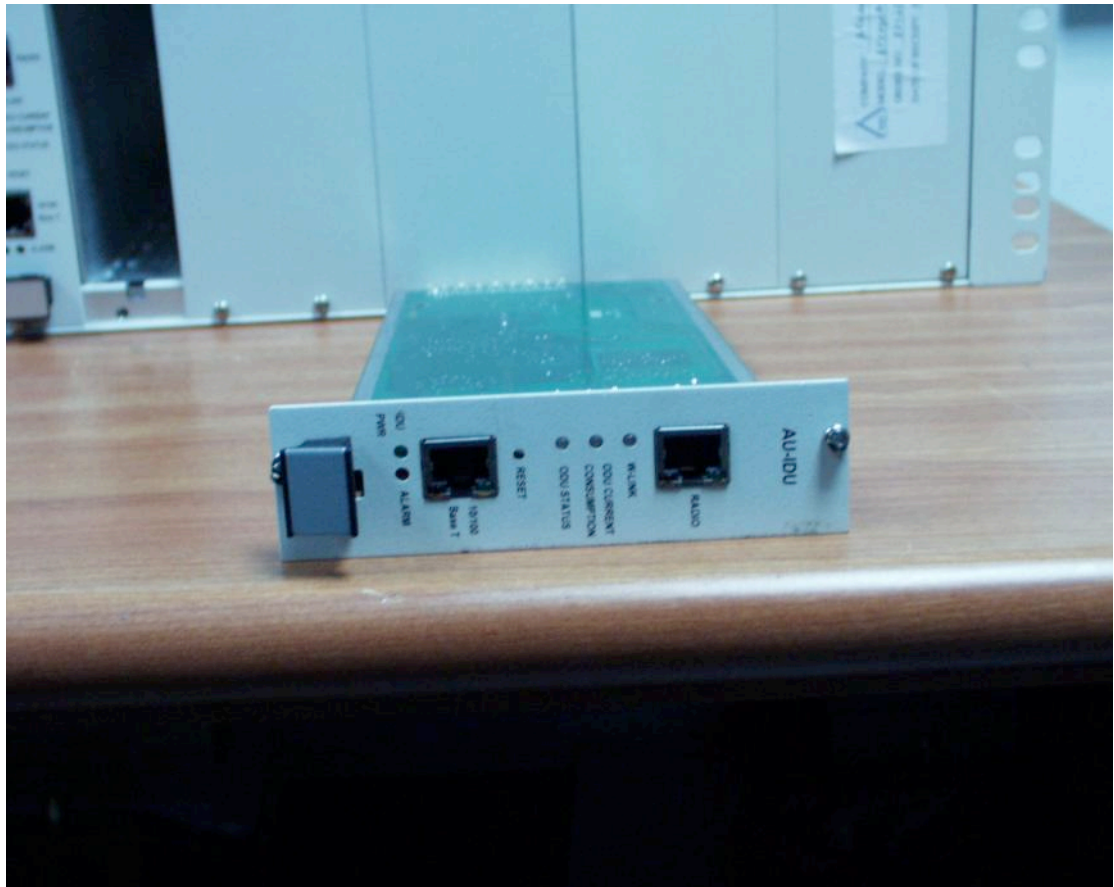
Base station indoor AU card, front panel
