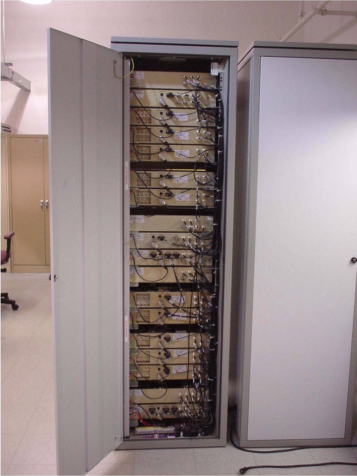
One Rack Rear View (with door open)
