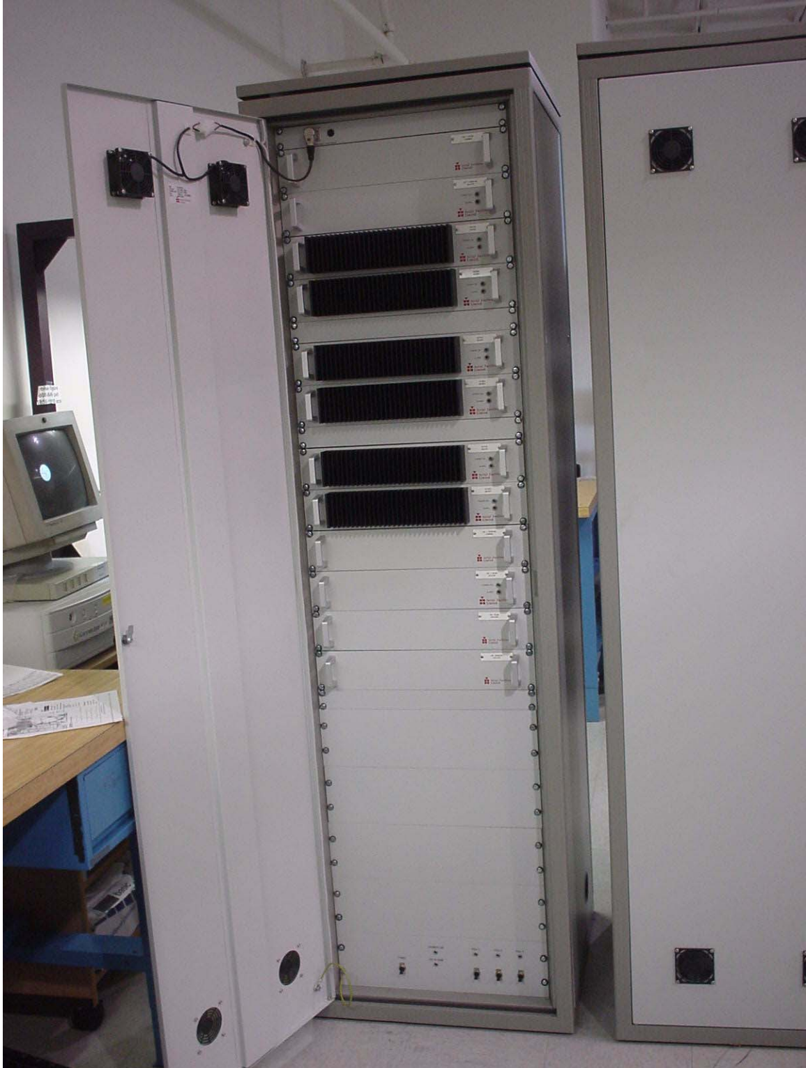
One Rack Front View (with door open)
