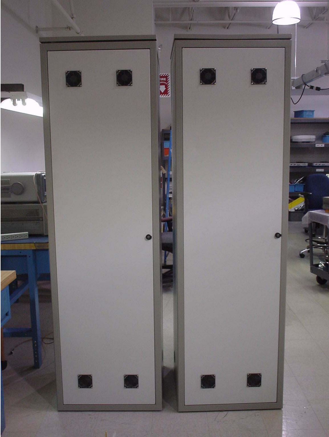
Two Racks Front View (with door closed)
