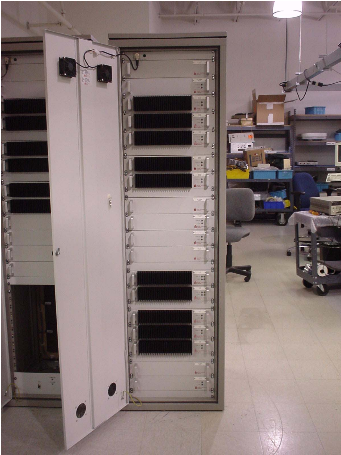
One Rack Front View (with door open)
