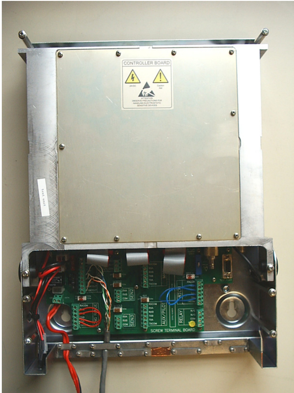
Photograph 4: MT-1 removed cover
