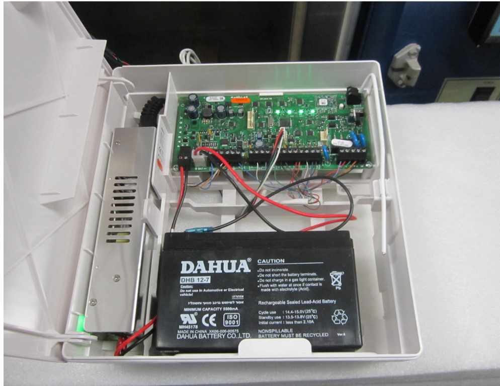
Photograph No.1 Wireless control panel board internal view
